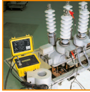
Measurement of the ratio on a current transformer
